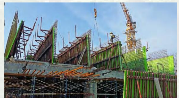
▲ Image shown Plasform in action at the construction site of a high rise condominium project at Merak Mas, Melaka.
