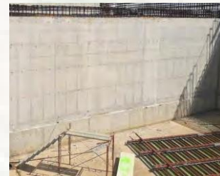
◀ Image shown a section of casted wall surface using Plasform, the surface is smooth and requires just skim coat to create a seamless finish.
